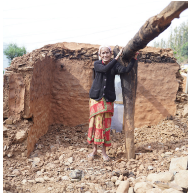
Shiladevi is standing inside her house damaged by the earthquake. ©Plan International
