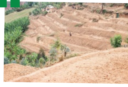
Radical terraces have been constructed on the arid mountain within the refugee camp.
